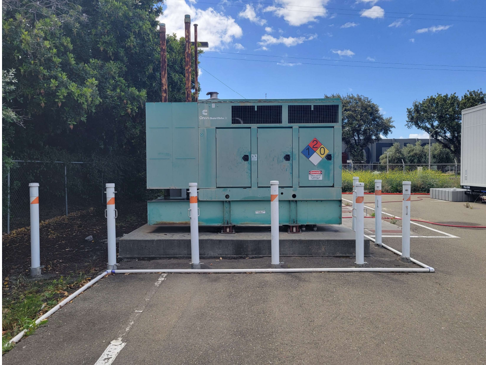
Backup generator serving temporary offices.
