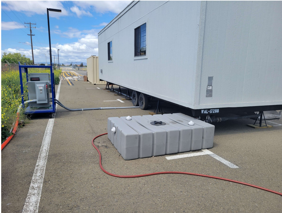
Water pump and sanitary storage tank associated with temporary offices.
