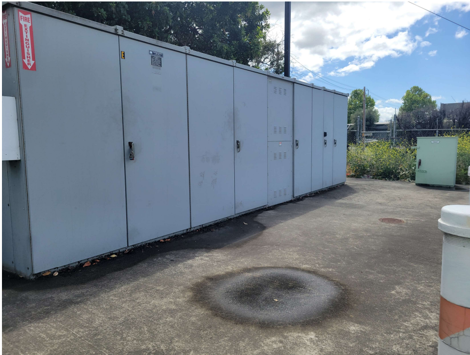
Electrical equipment associated with temporary offices.
