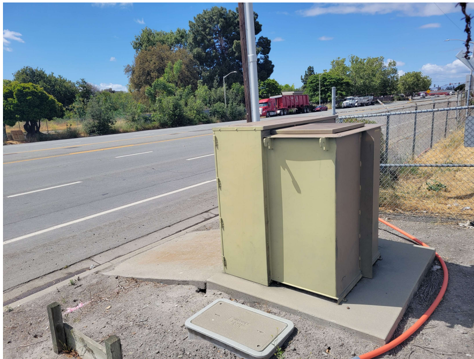
Pad-mounted transformer located near northwest corner of Subject Property.
