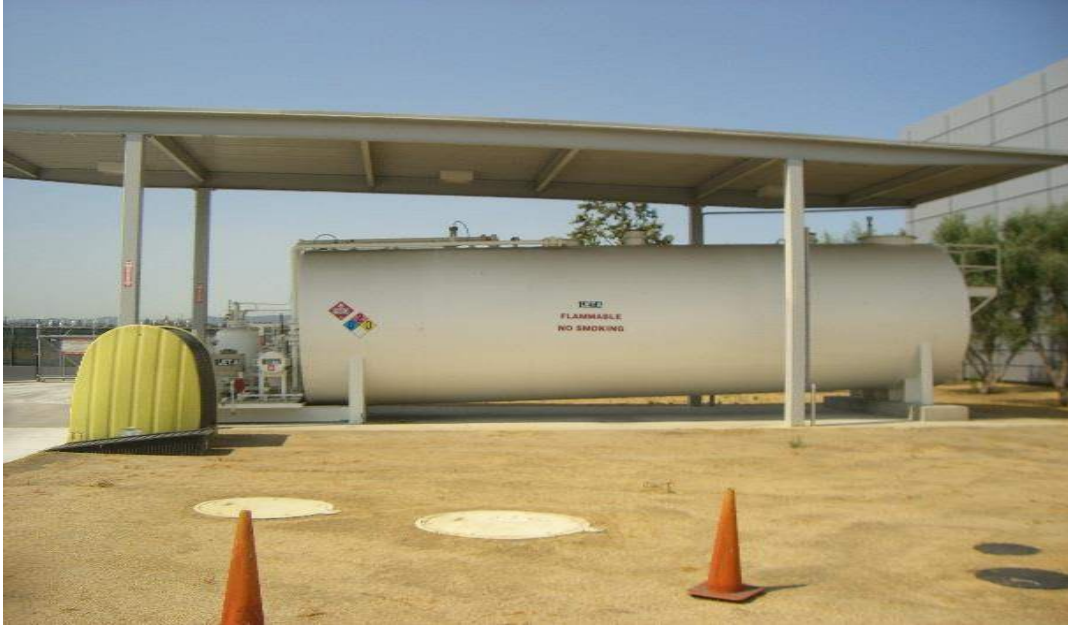
AVBASE ABOVE GROUND FUEL STORAGE TANK
