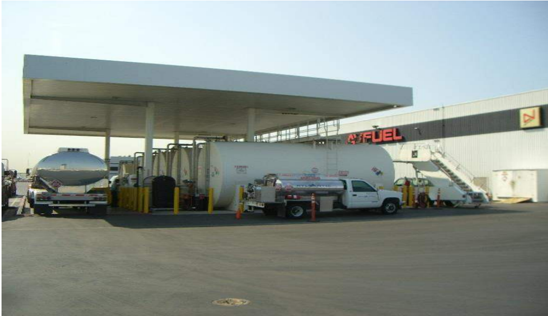
ATLANTIC AVIATION ABOVE GROUND STORAGE TANK FUELING RACK
