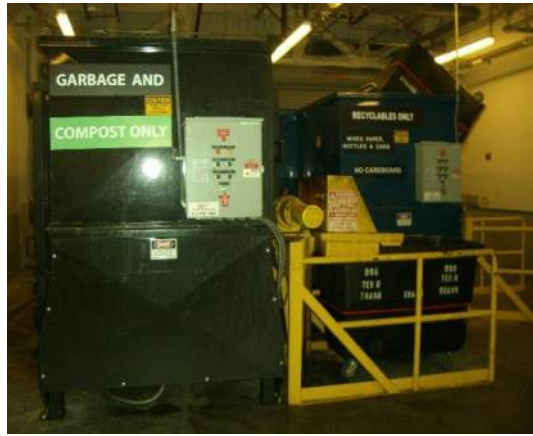
TERMINAL B COMPACTORS
